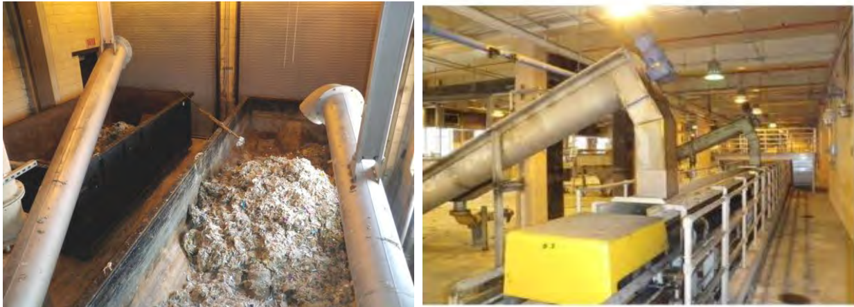
Figure 1: Grit Trailer (Left) and Grit Conveyors (Right) at Deer Island Wastewater Treatment Plant
