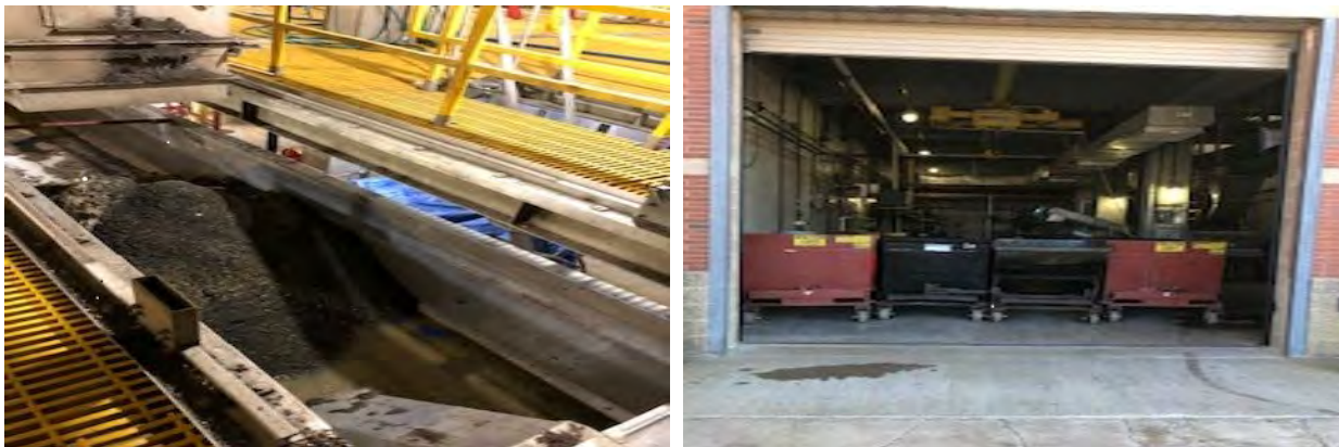
Figure 2: Grit Chute and Trailer at Nut Island Headworks Facility (Left) and the grit bay with Dumpsters at the Intermediate Pump Station (Right)
