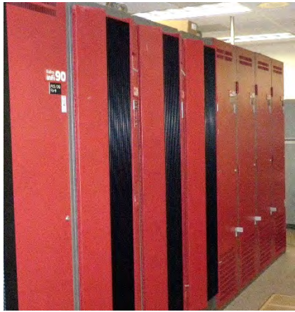
Figure 1: PICS DPU Cabinets
