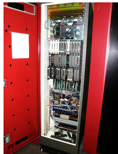
Figure 3: DPU Cabinet Showing Control Modules
